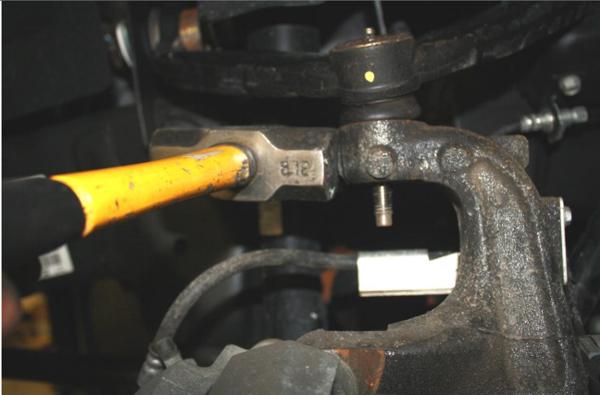
Figure 1: breaking ball joint loose from spindle
